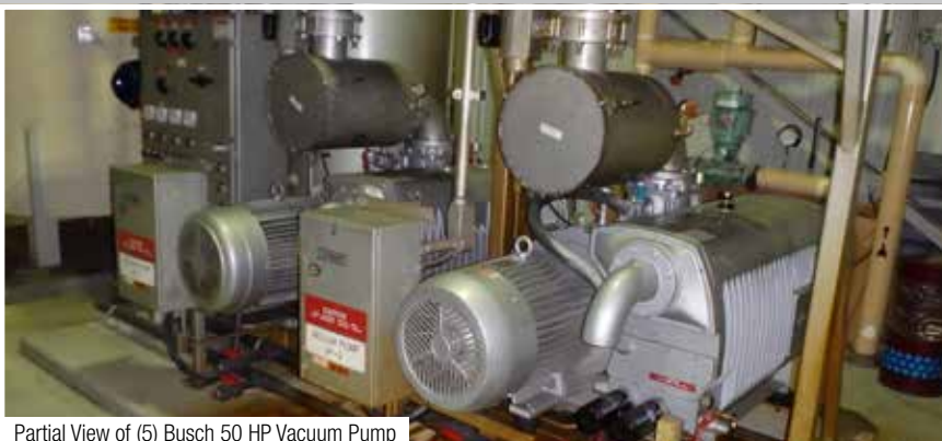
Partial View of (5) Busch 50 HP Vacuum Pump
