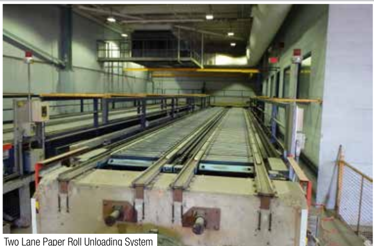
Two Lane Paper Roll Unloading System
