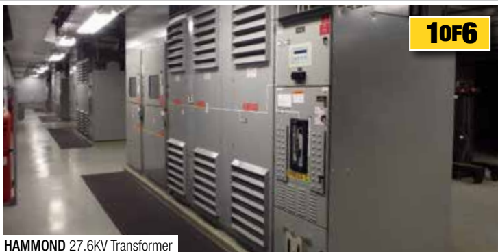
HAMMOND 27.6KV Transformer
